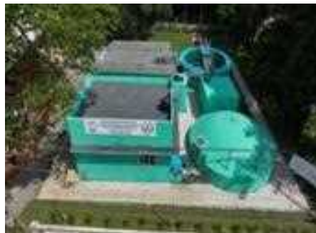
360 KLD STP at General Hospital, Thrissur
